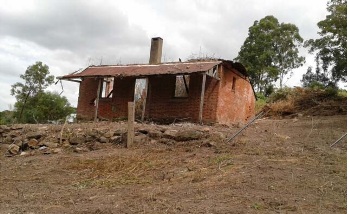
In 2016 vegetation was removed from around the cottage (photo by Val Patfield).
